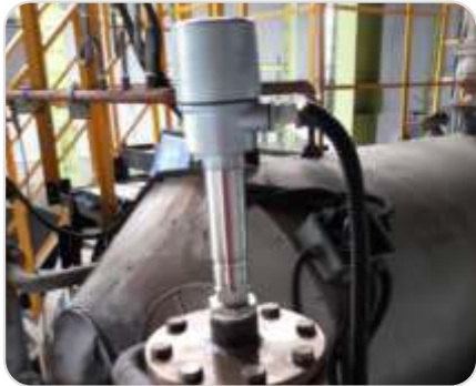
High temperature boiler
